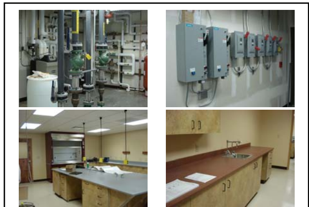
Bldg #8415 – Mechanical Spaces and Lab
