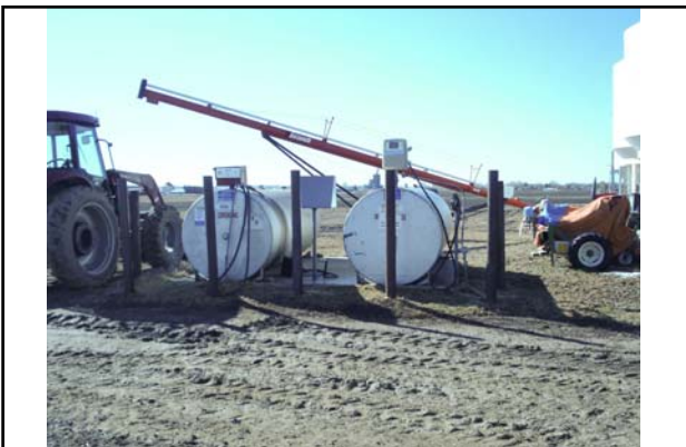
Bldg #8418 - Fuel Tanks
