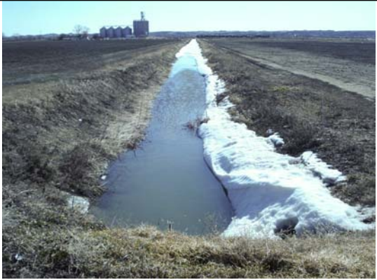
Canals will eventually need some work
