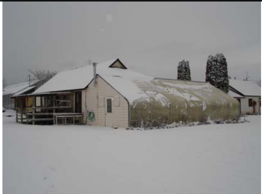
Bldg #7405 Grindhouse & Greenhouse (image is focused on the Greenhouse – right part of L-shaped building)
