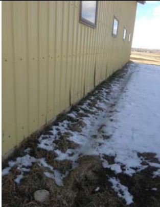
Damage siding from lawnmower
