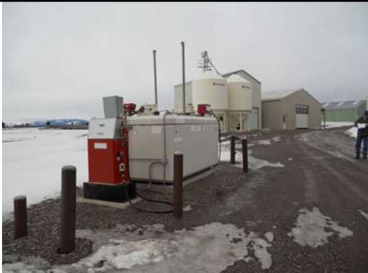
Bldg #760 - Fuel Tank (709, 727, & 704 also in picture)
