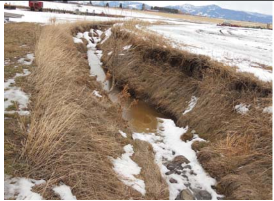
Irrigation Canal (Erosion Issues starting to occur)
