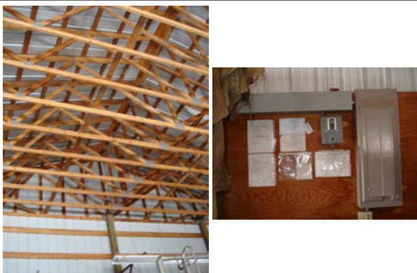
Bldg #6412 - Research Distillation Facility
