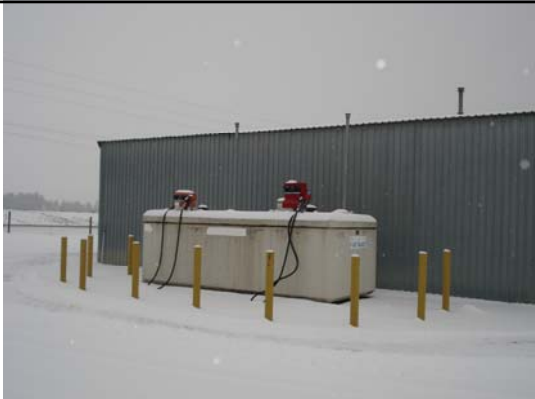
Bldg #6421 – Fuel Tanks
