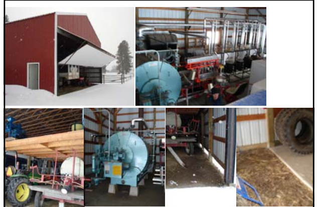
Bldg #6412 - Research Distillation Facility
