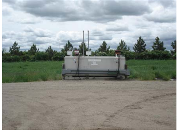
Bldg #5462 – Fuel Tank 1500 Gal
