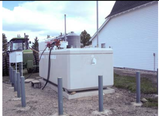
Fuel Tank on West Side of Bldg #4413
