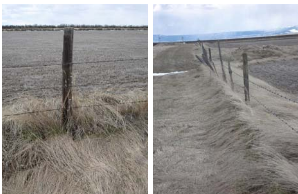
Fencing deteriorating, ground sagging near fence
