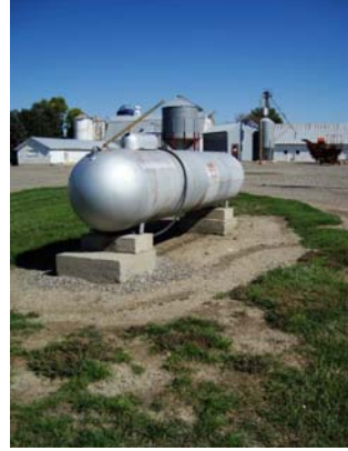
Unnumbered Propane Tank
