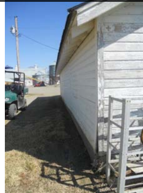
Bldg #3433 - Cereal/ Crops Lab - Wall is warping due to settling foundation
