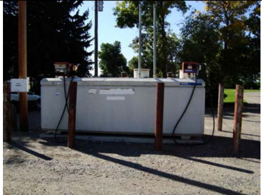
Gas Pump close to Truck Scales
