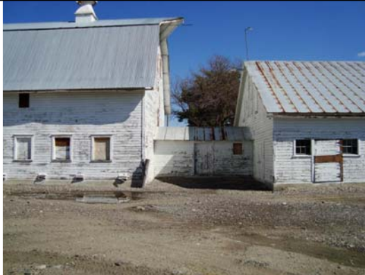
Connection between bldg #3465 condemned section of Barn Complex and #3421 Southern Annex of the Barn Complex used for storage
