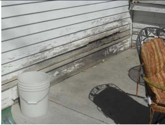
Bad siding on bldg #3404 – Residence
