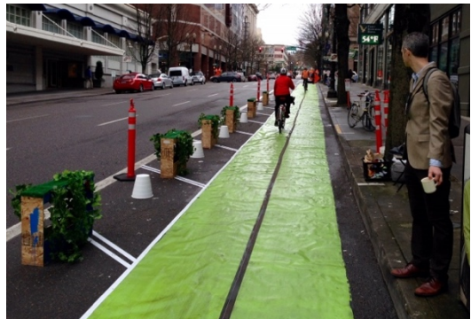
Figure 6: The use of temporary paint and chalk may look similar to what is shown in this photo.
