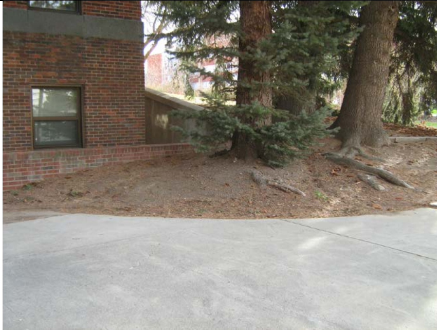
View of brick retaining wall, concrete retaining wall with concrete cap and exposed tree roots.
