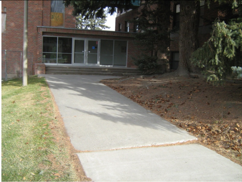
Sidewalk to the entrance at the connecting corridor between Cooley and Lewis is heaving and sinking in numerous areas.
