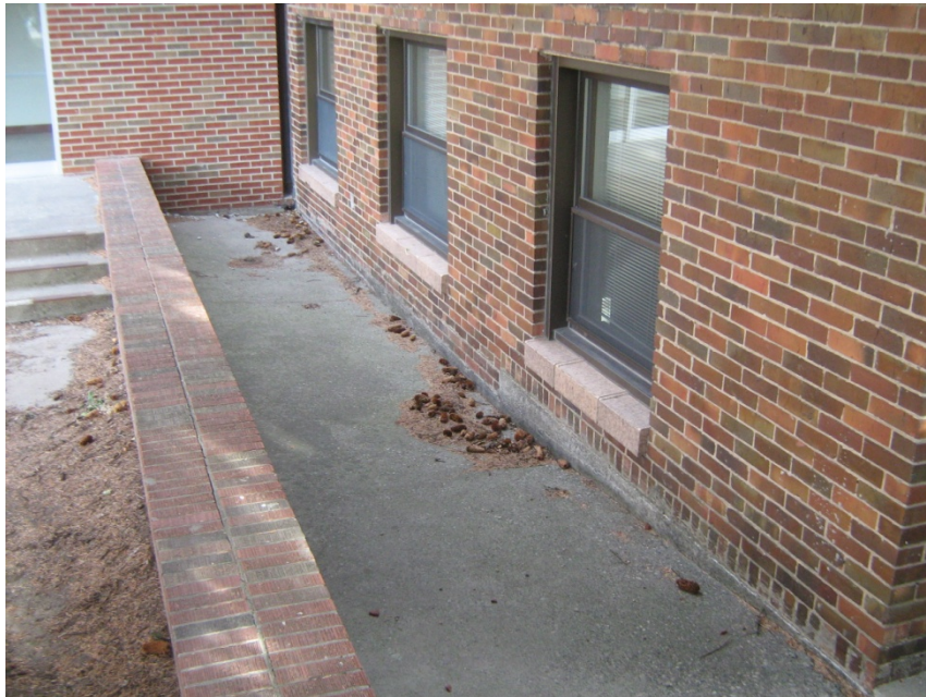
Area drain west of Lewis. The concrete pad, brick wall, and steps are in poor condition.
